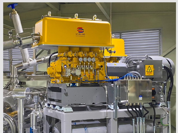
200 kg/day hydrogen boil-off gas re-liquefaction system as part of a large liquid hydrogen facility at a Korean Institute (2025)
