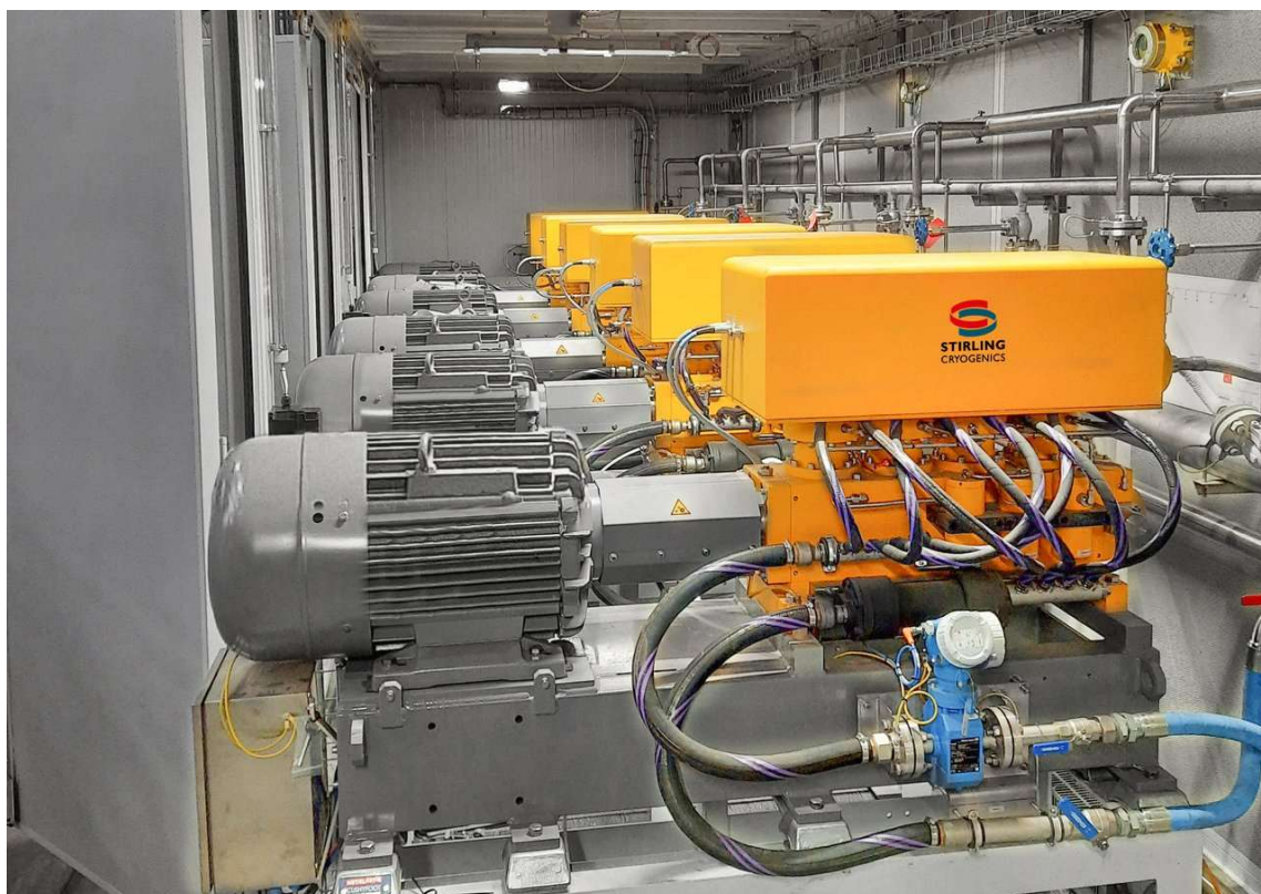
Containerized liquefaction system
